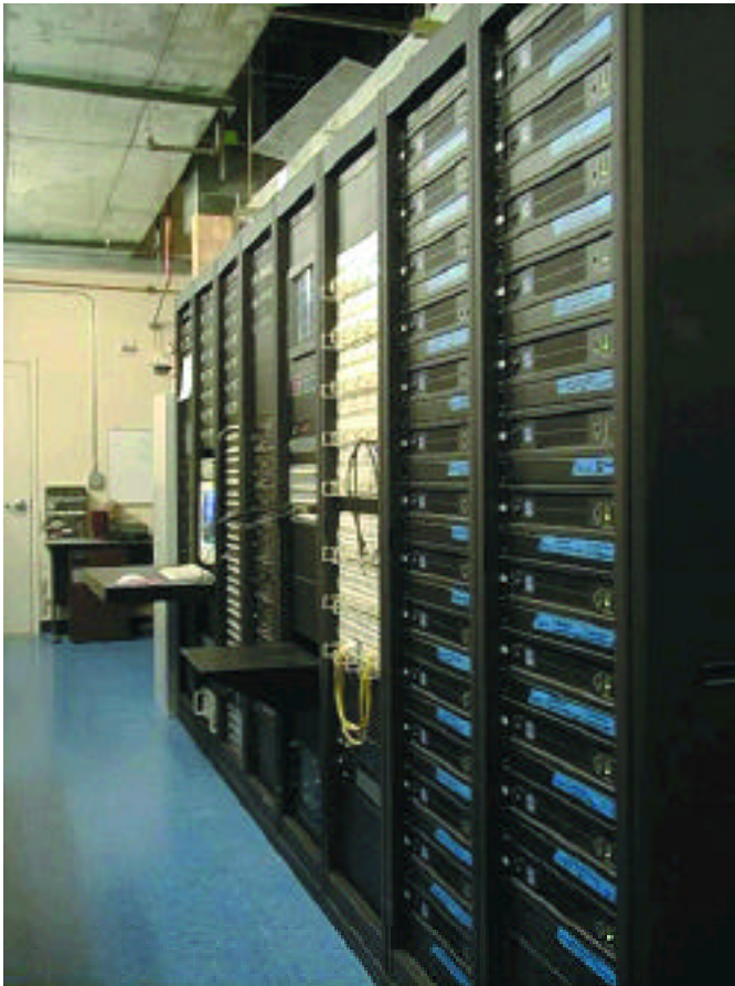
'Patch Central' in the Aladdin Conference Center A/V room provides effective access to over 1500 tielines.
