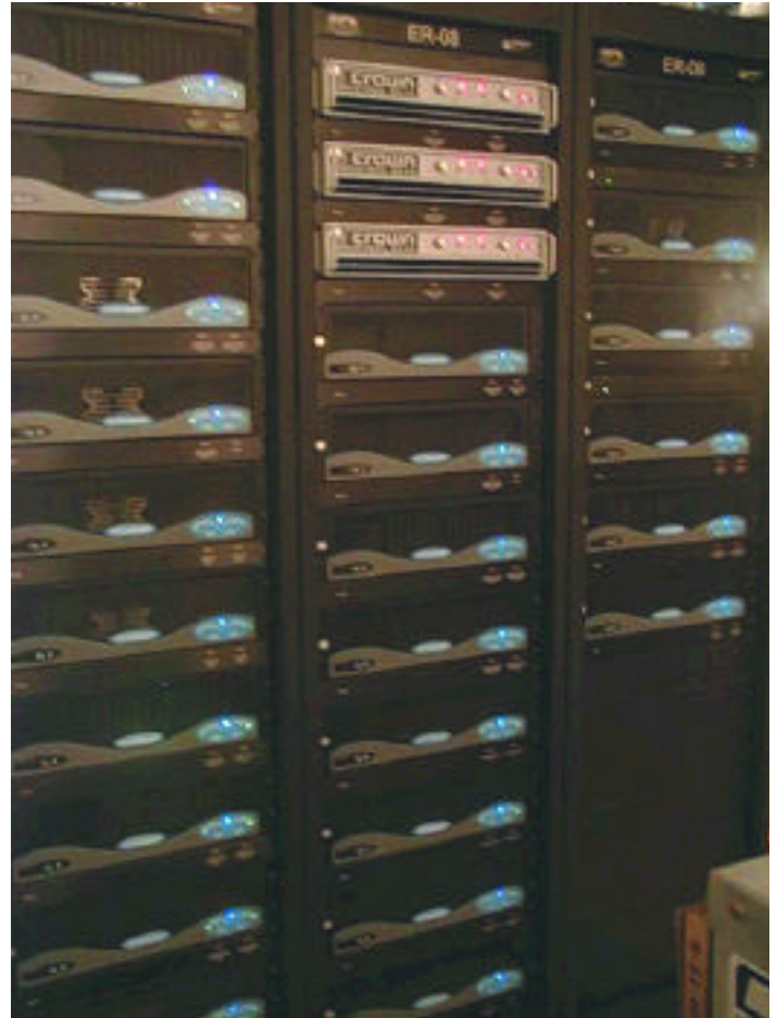
SPL showcases the Crown Contractor series amplifiers in the amplifier's debut installation in the Aladdin BGM system.
